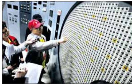
Visitors can see powerful computers – the most advanced in the 1980s – in the central control room.
