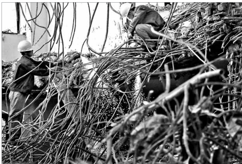
Construction workers cut iron bars to make way for new residential and commercial spaces where Taiwan Hotel used to stand. IC Photo
