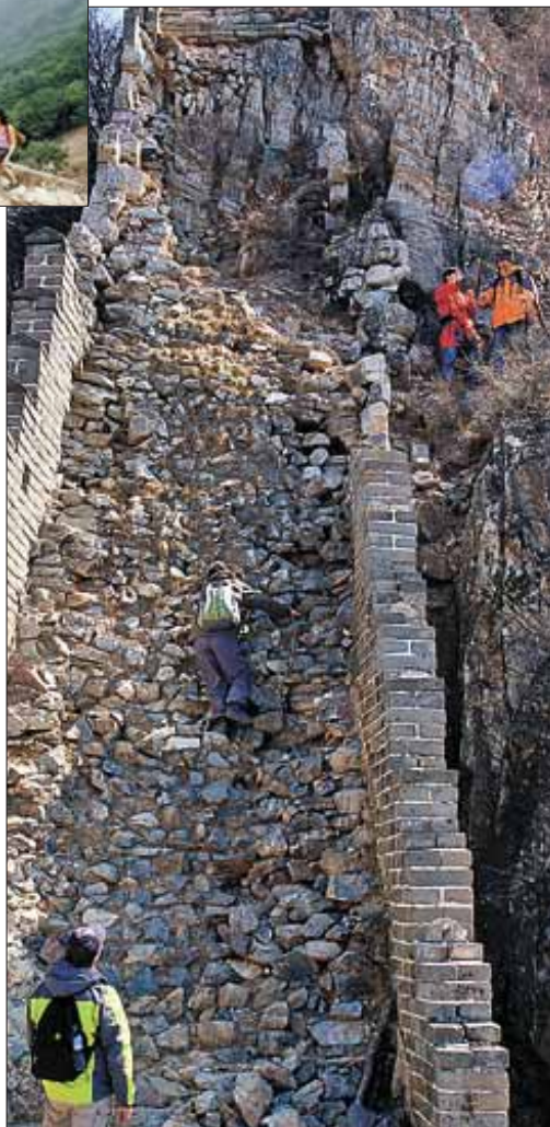
The stairs on the Jiankou Great Wall are badly destroyed.
